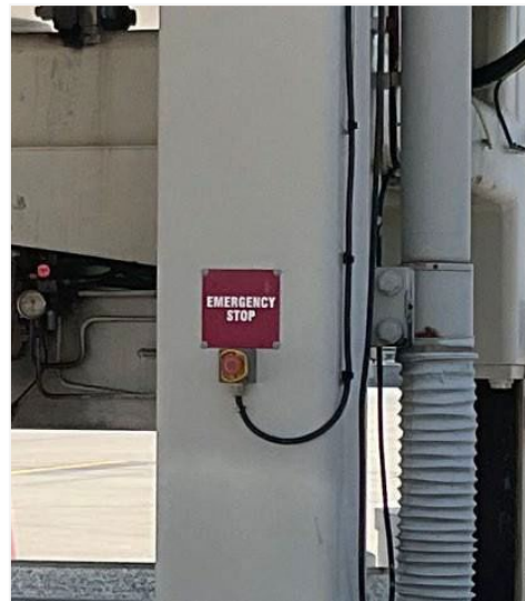
Figure 26 Aerobridge Emergency Stop Button
