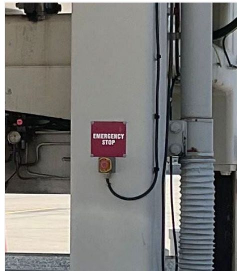
Figure 26 Aerobridge Emergency Stop Button
