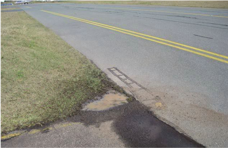
Figure 31 Example of leaving paved areas resulting in mud, grass and gravel on taxiway
